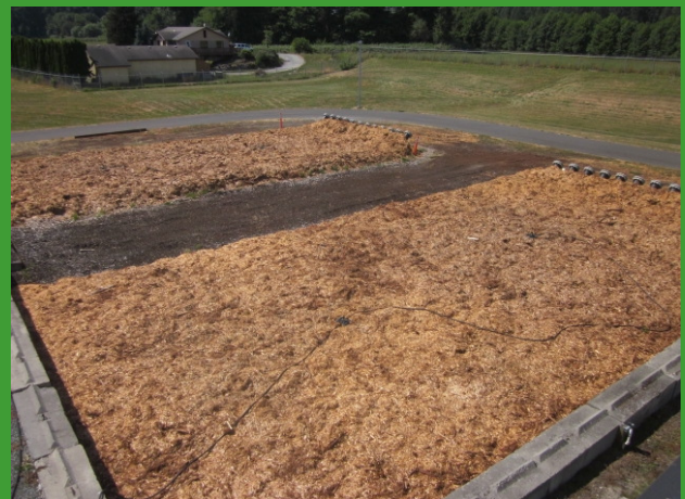
Bio Filter Beds at the Wastewater Treatment Plant
