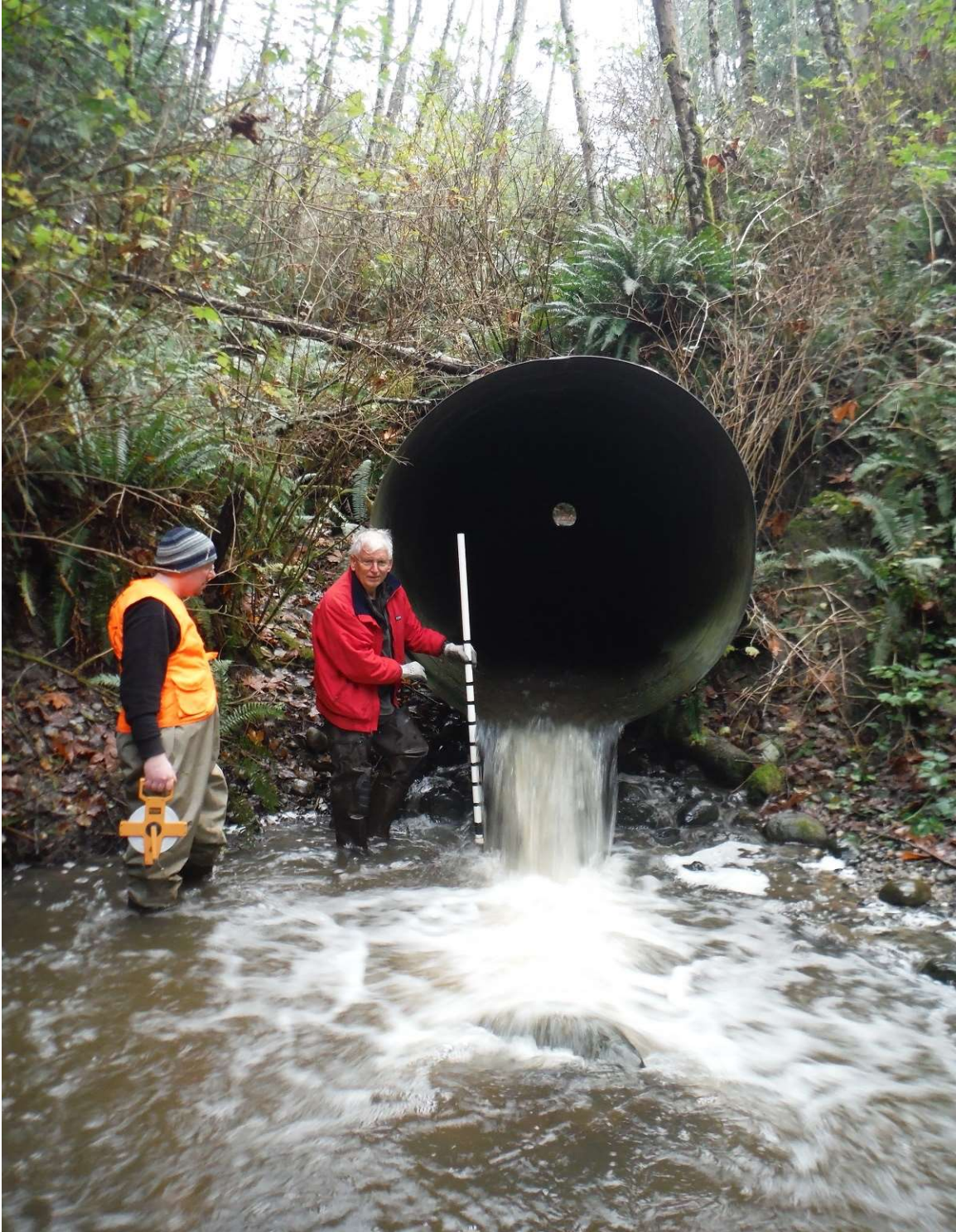
2016 6 ft.. diameter, 210 feet long culvert, steep, a mess, and total fish passage barrier.
