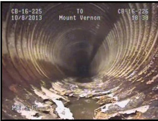
Rusted out Corrugated Metal Pipe (CMP) in need of lining or replacement
