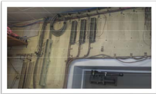
Evidence of diesel soot is shown in this picture
