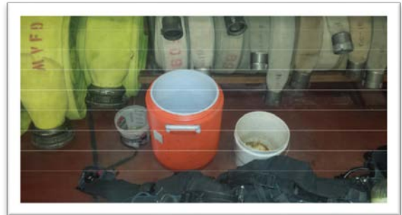
Strategically placed buckets and containers catch water dripping from roof leaks so firefighters don't slip in puddles
