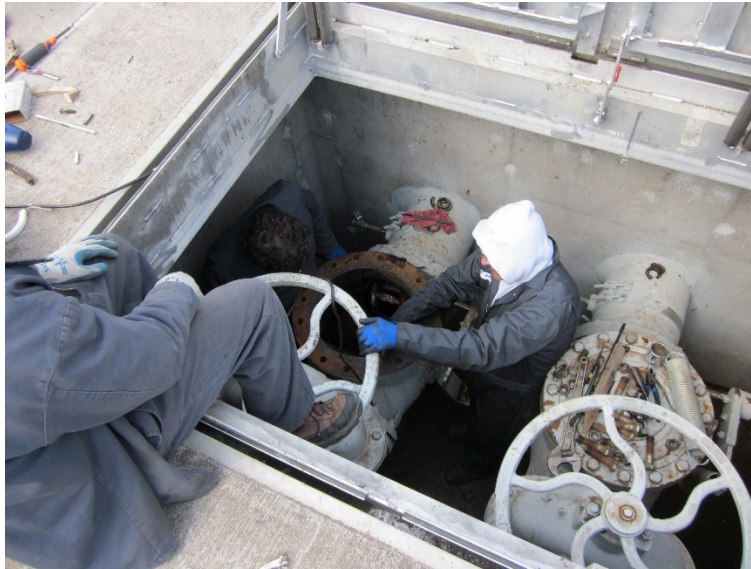
College Way Check Valve
