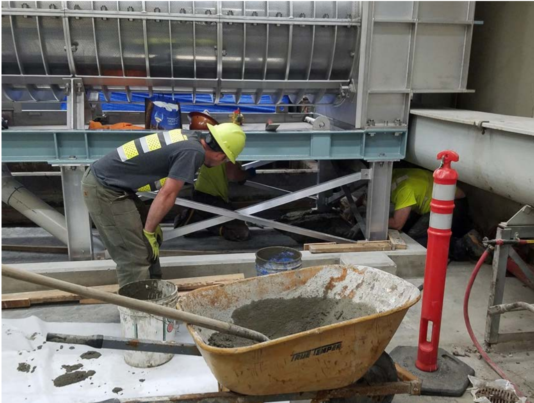
Biosolids Screw/Rotary Press Installation
